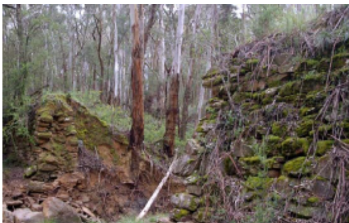
Above: Eaton's Dam showing the flood damage from 1933.
